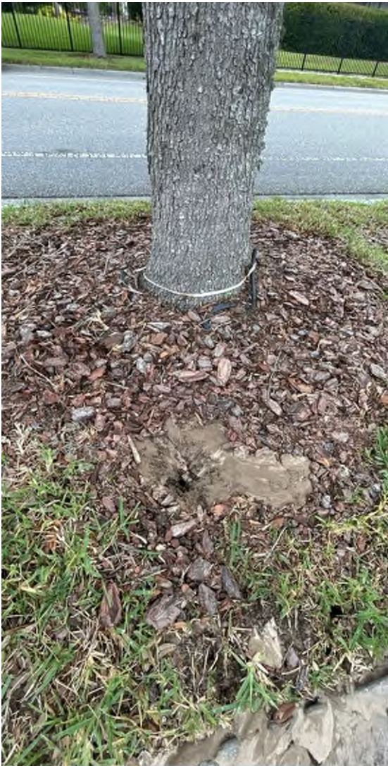
M36 lateral leak
